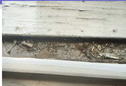
Lead paint cracking, and chips in a window well. Photo—Sara Kerley
